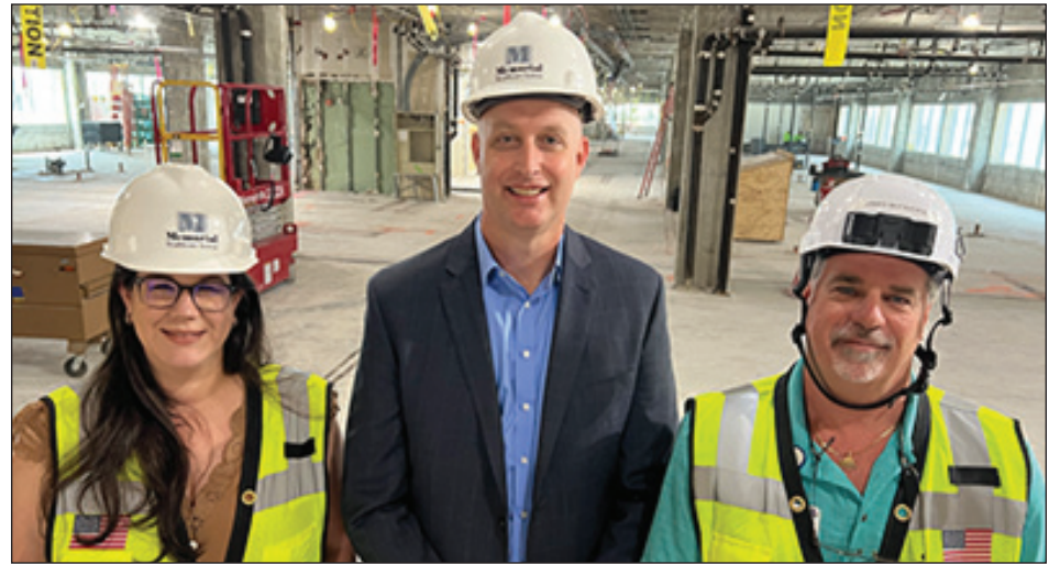
Marta McNab, Jon Pickett and James Mcfadden in the Family Birthplace construction site.
